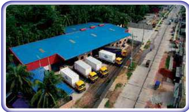
CNG Compressor Station at Bhola
